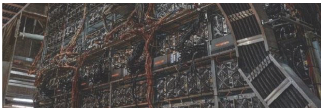
Bitcoin mining equipment installed within the Town of Torrey, NY mining facility.
